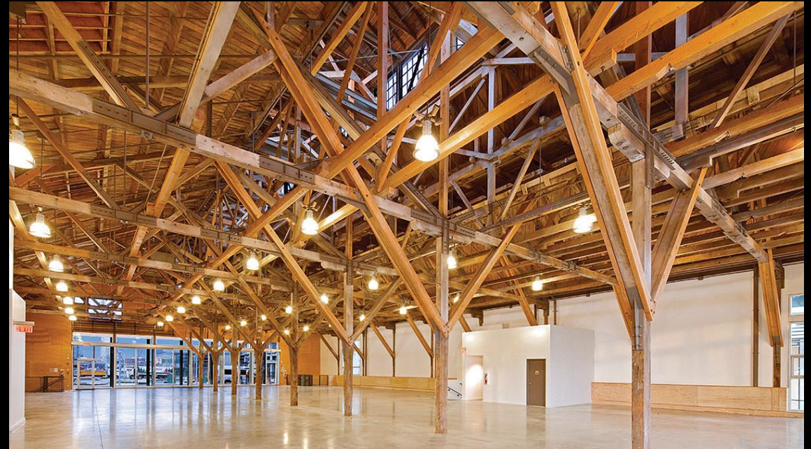
Timber trusses were repaired installing steel plates at connection points, credit: Acton Ostry Architects
